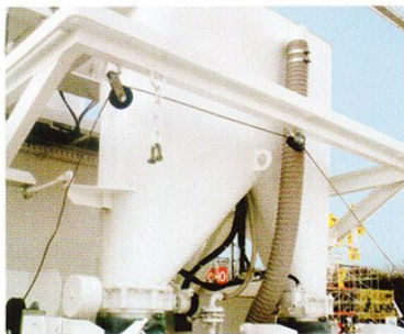
Cement and water weighing system
